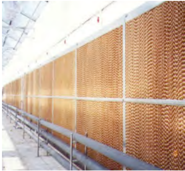
Water wall in the green house
