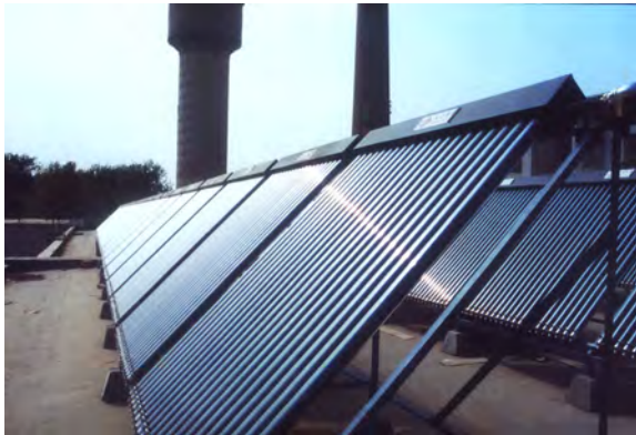
Figure 3.4.1 Solar water heater application on rooftop
