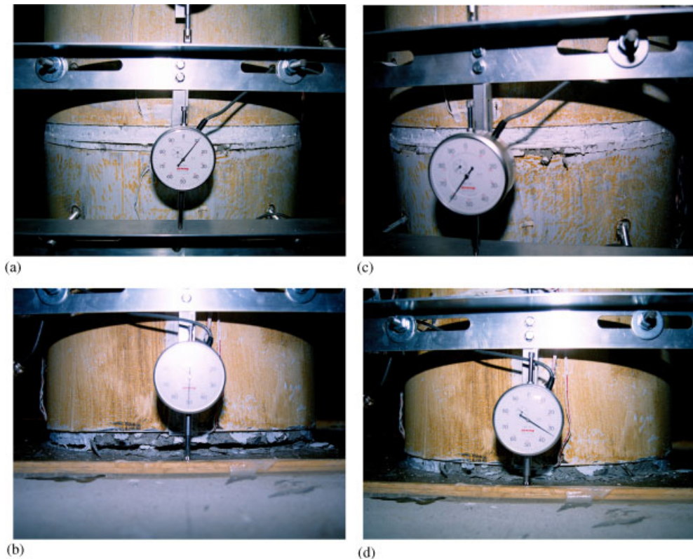
Figure 5. Specimen 1 at 4% drift: (a) opening between segments 1 and 2; (b) opening at base; (c) spalling between segments 1 and 2; and (d) crushing at base.
