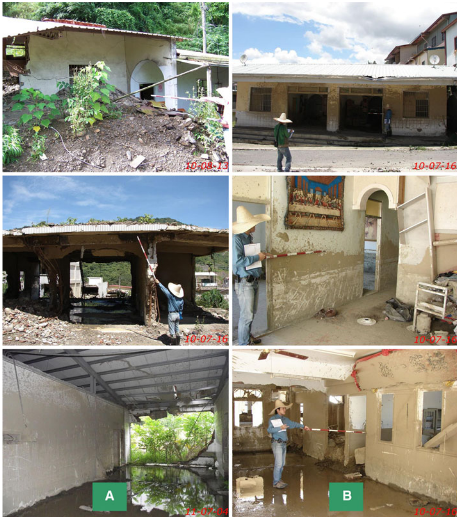
Fig. 8 Examples for structural damage assessed during field investigation: a when inundation height is \geq 2 m, and b when inundation height is < 2 m
