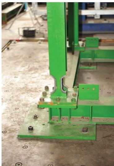
FIGURE 7: Flange partially cut out near the bottom of column.
