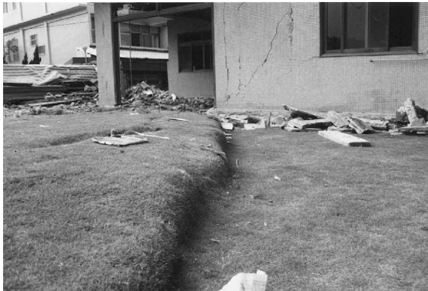
Fig. 23. Buildings in the uphill of village where rupture-B passed through were severely damaged.
