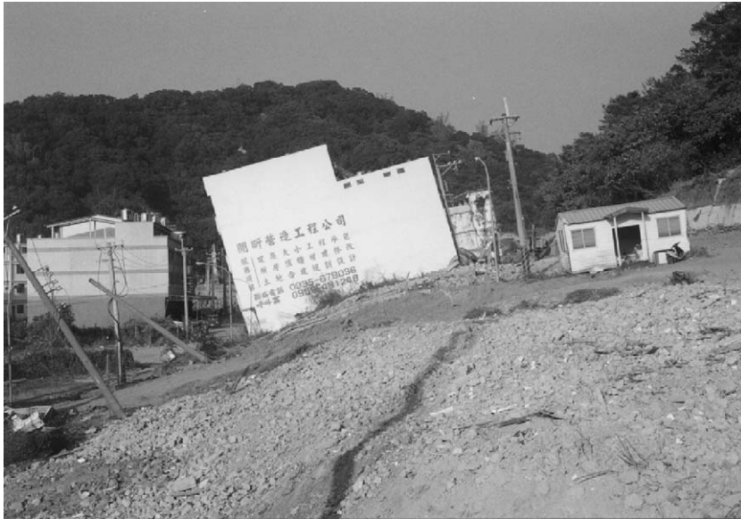
Fig. 20. Building in the center of the photo was tilted by uplifting of the hangingwall, but the structure remained intact.
