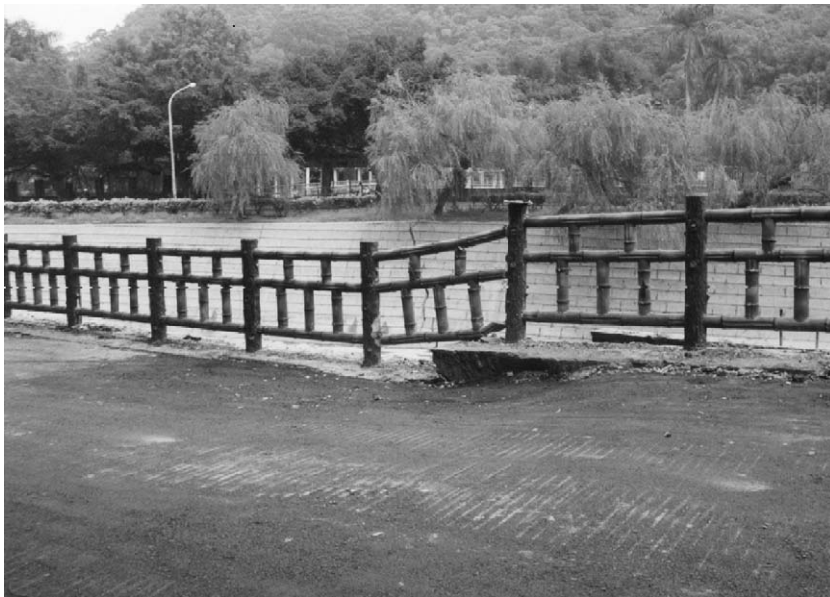
Fig. 6. Rupture-B near the Chung-Cheng park. Rupture-B lies between the main rupture and rupture-A. The vertical uplift of the surface rupture is 0.1–0.2 m. The east side of the surface rupture is higher than the west side.
