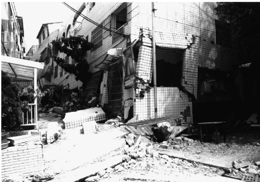
Fig. 21. Building on the hangingwall is damaged while the one on footwall remains intact.
