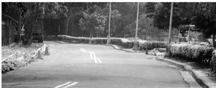
Fig. 4. The wavy road surface due to hangingwall deformation near the Chung-Cheng Park.
