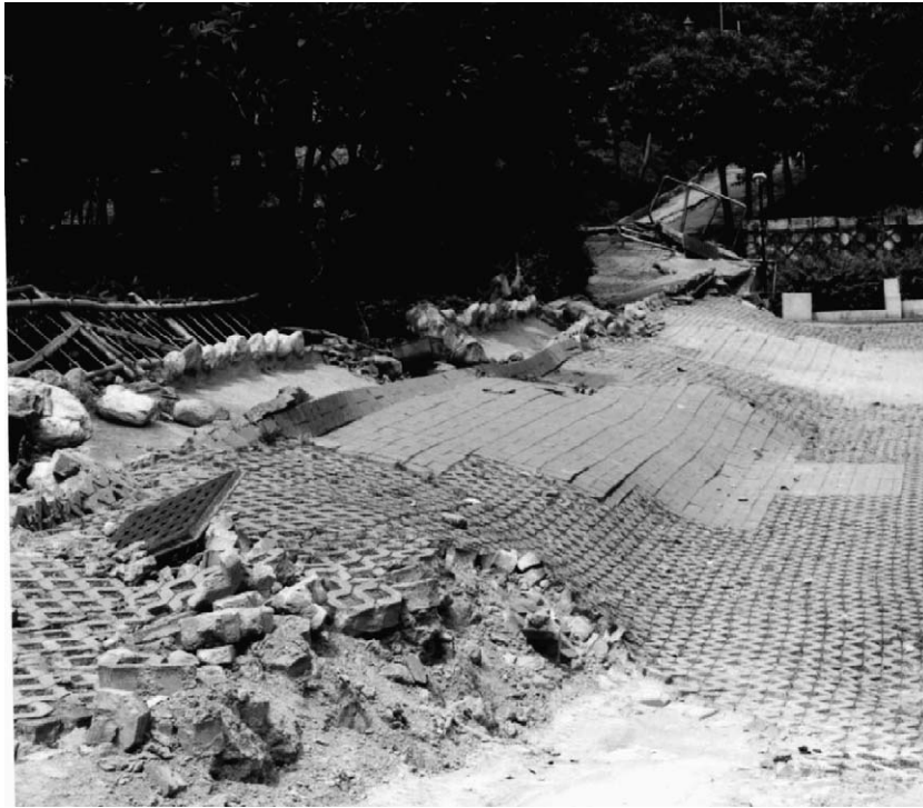
Fig. 5. Rupture-A in the Chung-Cheng Park. The left side of this photo faces west. The vertical uplift is 0.9 m.
