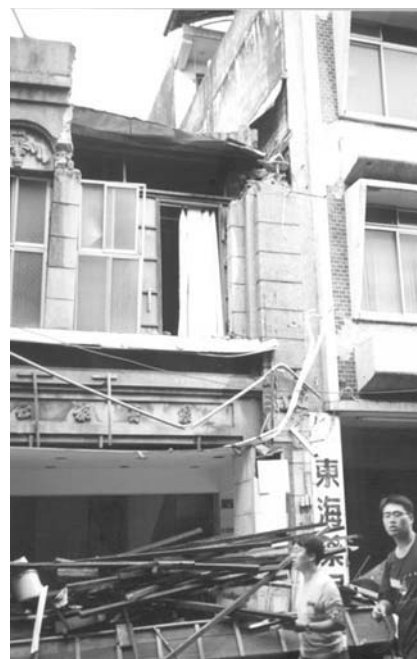
Fig. 3 Major damage example of structural pounding in Pu-Li
