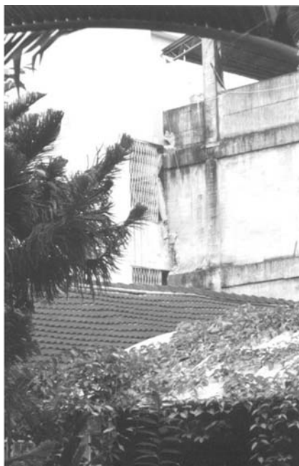
Fig. 4 Minor damage example of structural pounding in Dong-Shi
