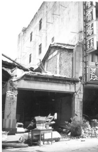
Fig. 2 Collapse example of structural pounding in Dong-Shi
