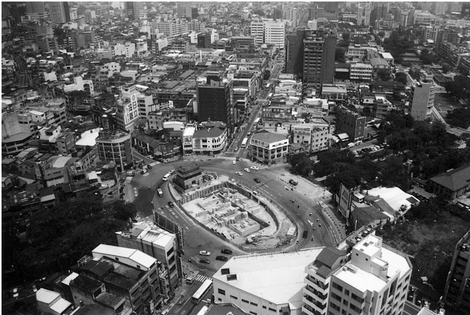
Fig. 7. The Plaza which is under construction and expected to be completed by the end of September, 1999 (photo by Jia-Chen Lin).
