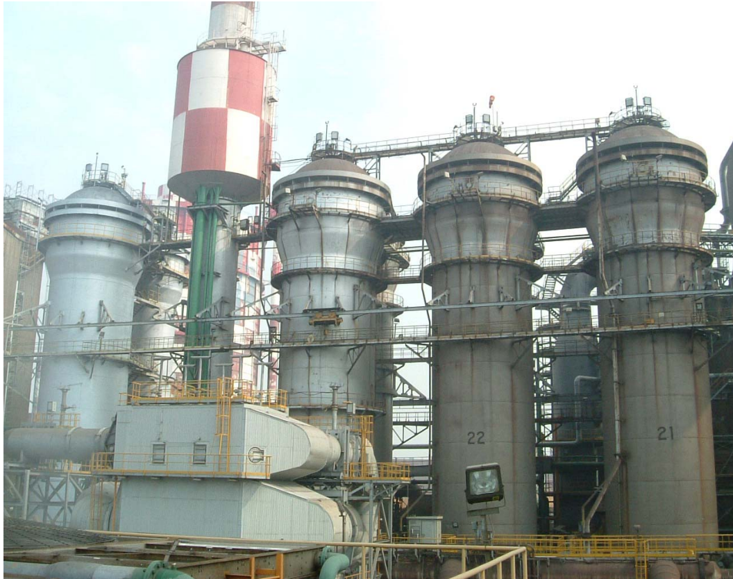
Fig. 2-1 Hot-blast stove of the China Steel Cooperation
