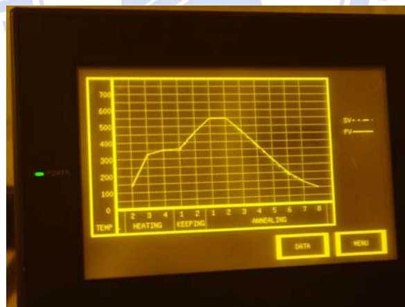
Fig. 3-13. The photograph of the temperature profile of the furnace.
