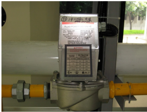
(a) Emergency shut-off valve
