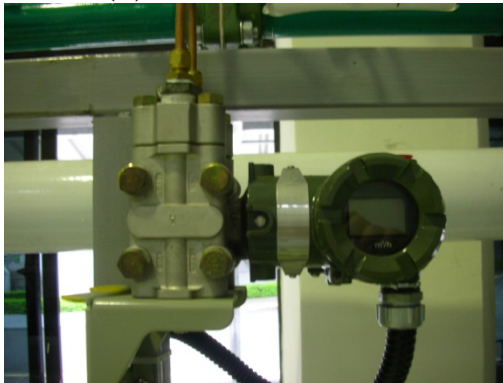
(c) Differential pressure transmitter
