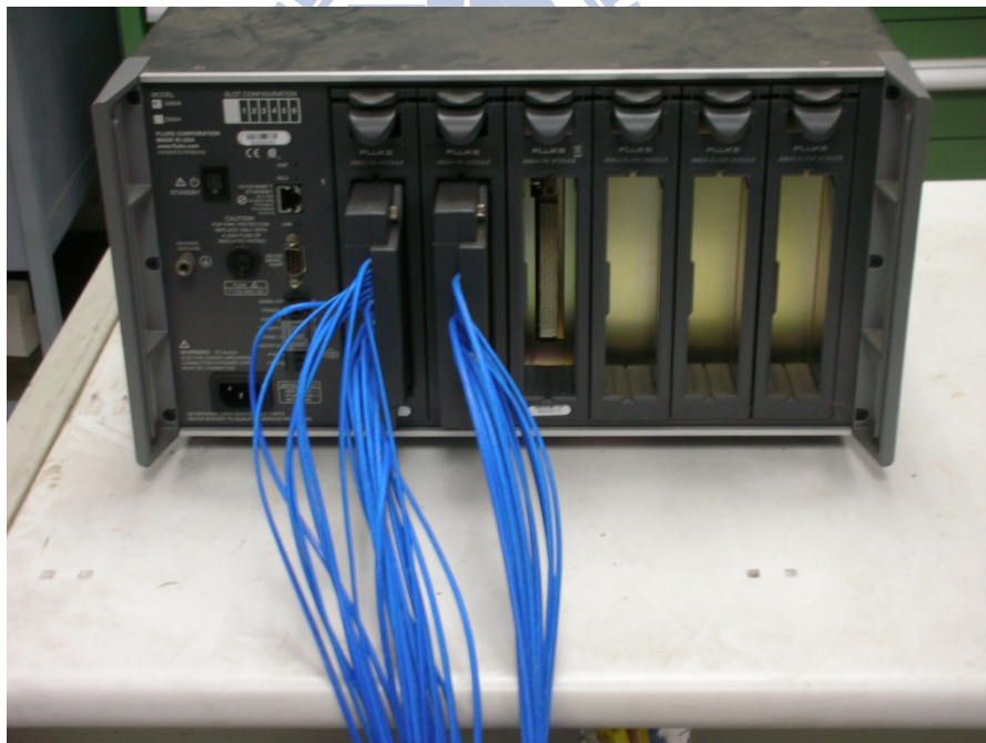
Figure 2.23 The picture of data acquisition system (Fluke 2680A Series) (a) Front view and (b) Back view
