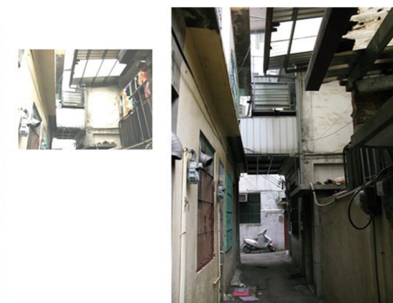
2. On the first floor is clear corridor, construction of additional floor above
