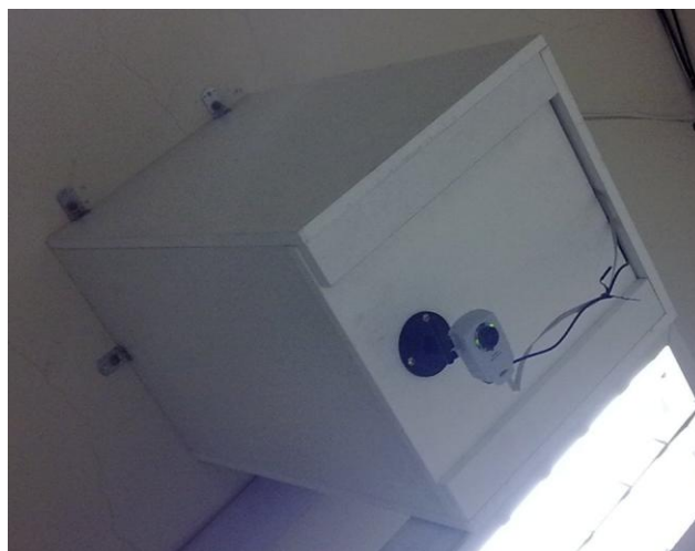
Figure 2.3 An Axis 207MW camera is affixed on the ceiling.
