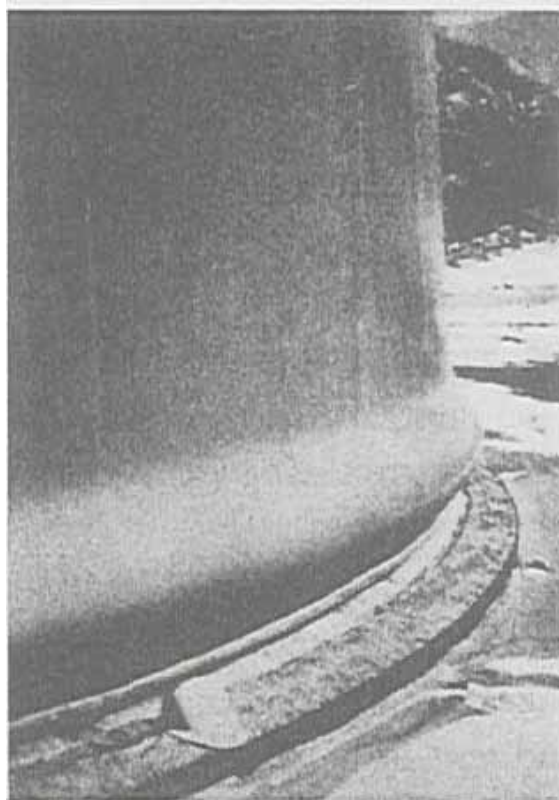
圖 1.1 槽殼挫屈 1971 San Fernando Earthquake, USA
