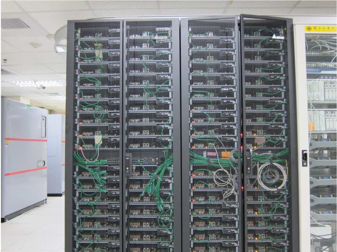
Figure 3.20: Servers and racks donated by Delta, Inc.
