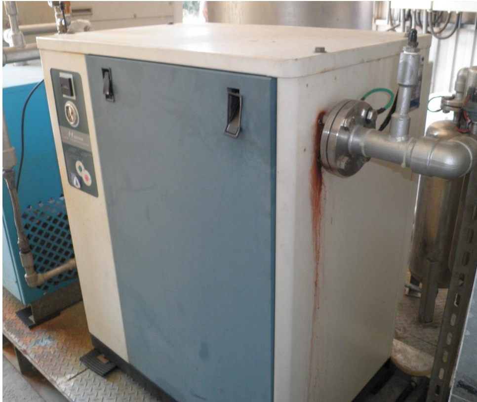
Figure 3.6 Air Compressor (H-50)
