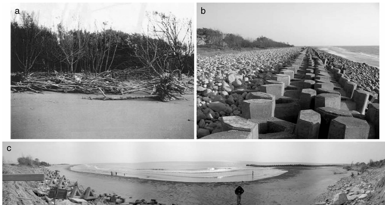
Figure 3. Photos showing the beach erosion at Kangnan Coast (a) before the construction of the breakwater (1998) and (b) after the construction of the breakwater (2000); (c) terminal scour at the end of the constructed breakwater (2005). For a color version of this figure, see page 397.
