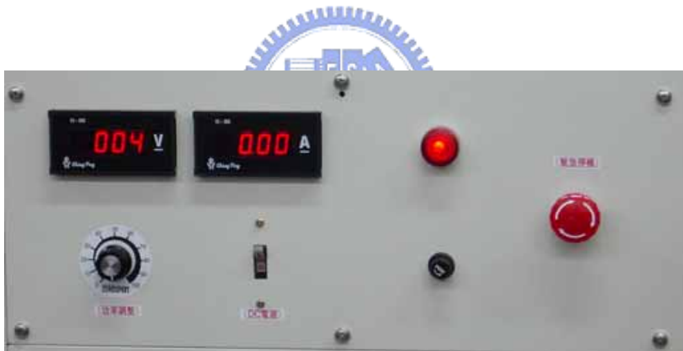
Figure 2.10. The DC power control panel
