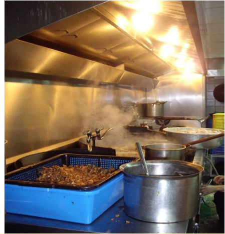
U-1廚房瓦斯器具未設置漏氣遮斷閥
