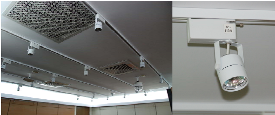
Figure 6.5: UPnP-enabled whole lighting devices.
