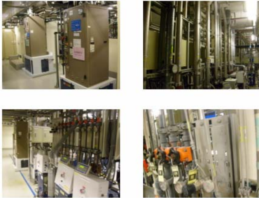
圖 1-1 CVD Utility 區主要設施為:PUMP (Line)、Local Scrubber
