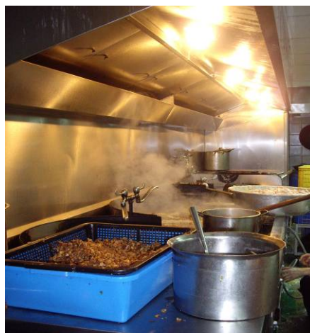
B1廚房瓦斯器具未設置漏氣遮斷閥
