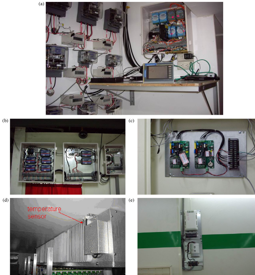
Fig. 10. The convenience store energy management system: (a) overview; (b) 220 V power meter and DIO module; (c) 110 V power meter; (d) low-temperature sensor in combination case; (e) indoor temperature, humidity, CO 2 , and illumination sensor.
