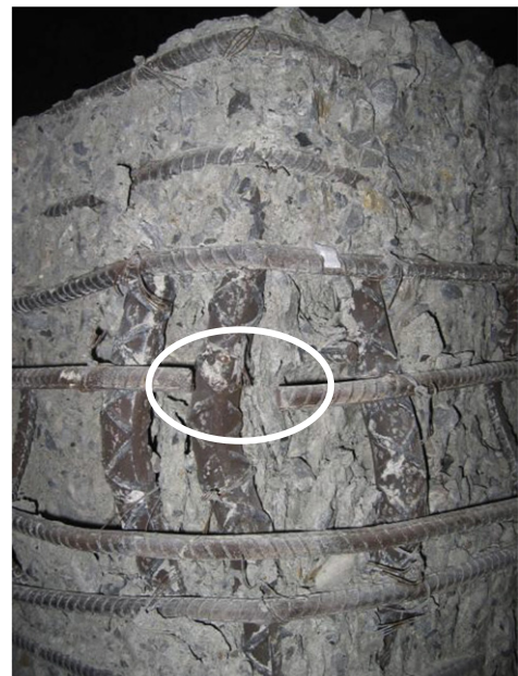
Fig. 9. Fractured rectilinear hoop and buckled longitudinal bars in the specimen DH-TI-90.
